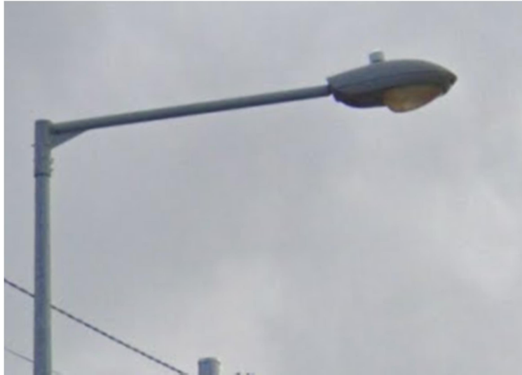
Figure 4-3 150W Metal Halide Light
