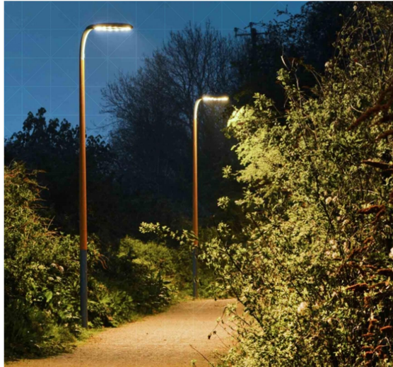
Figure 4-8 Pedestrian Walkway Lighting
